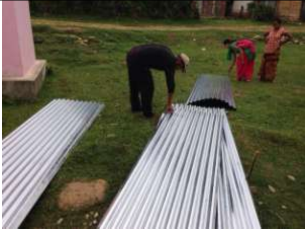
New iron sheets for repairing roofs being done by SADP Nepal in Tanahu district in Nepal with funds donated by individuals in Canada, June 2015. Photo courtesy of S. Dahal.
